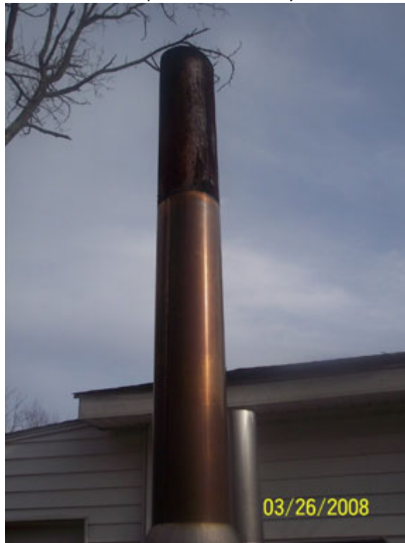
This is a picture of the chimney with an added piece to get the chimney above the garage roof.
