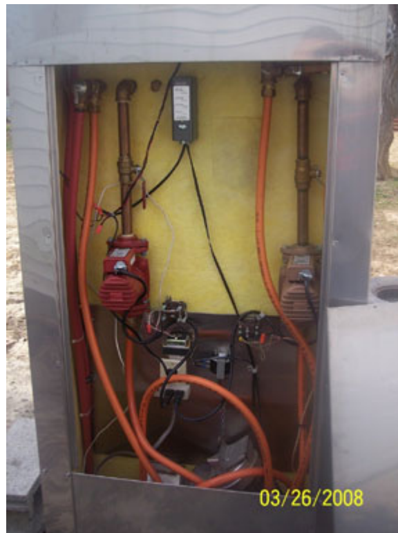
This picture shows the backside of the Hardy H-2 with the back panel removed. The thermostat, two pumps, blower, and hot water tank feeds.
