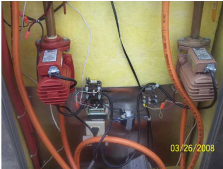
This picture shows the two pumps. The red pump feeds the house furnace and the brown pump feeds the garage heat exchanger.
