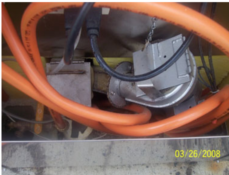
This picture shows the blower.
